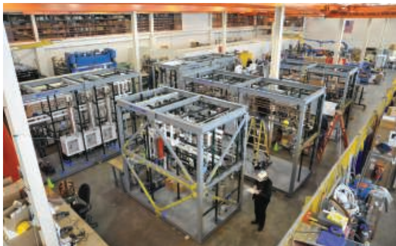
FIGURE 4. 'Cold eyes' reviews can assist in making larger pilot plant and research projects proceed more smoothly, allowing issues to be addressed and rectified earlier
