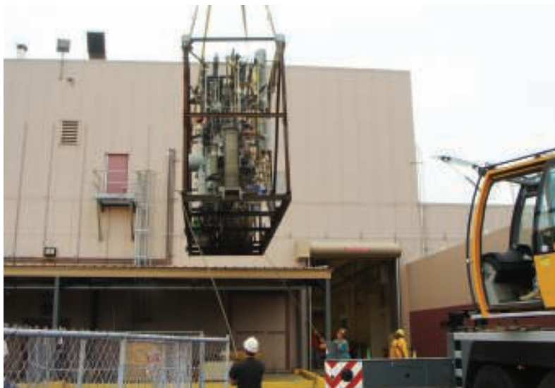
FIGURE 2. All projects have different critical steps and a good 'cold eyes' review will help the team to focus on the most critical ones
